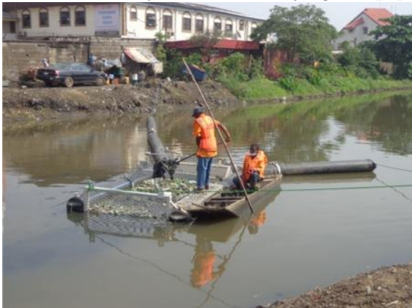
Movable Waste Screen @ Alaka Canal
